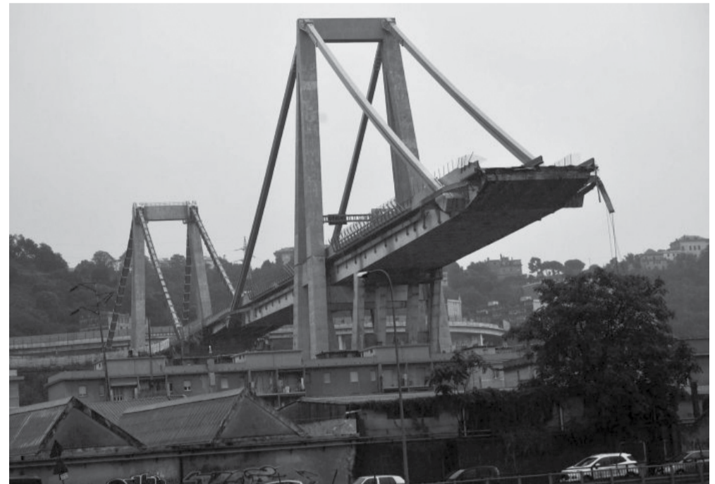
Ponte Morandi after its collapse in August 14, 2018
